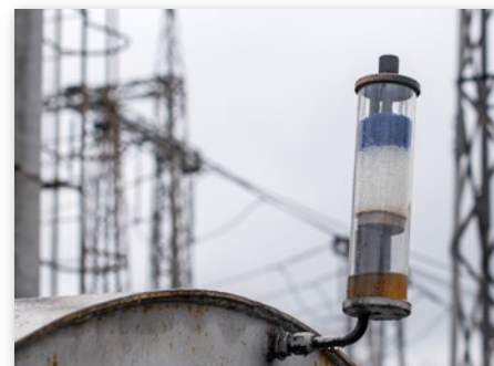
Fig. 1: Insulating oil used in transformers must be tested regularly.
